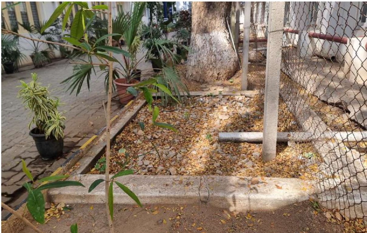
The rain water harvesting unit
