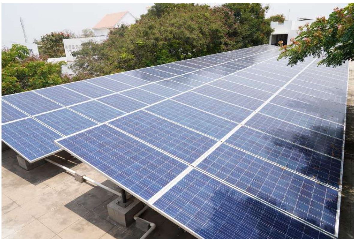
Solar roof panels in the college campus
