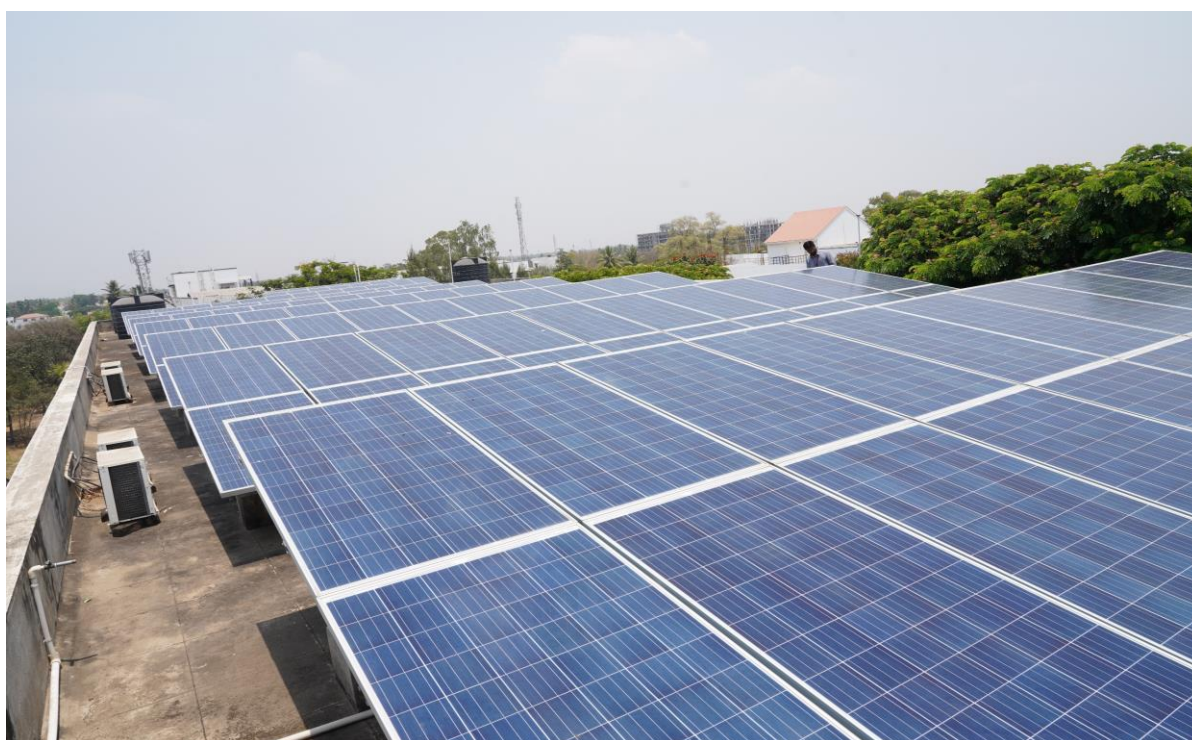
Solar roof panels in the college campus
